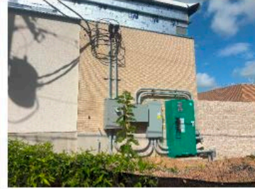
Permanent power now on
