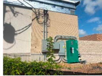
Permanent power now on
