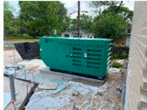
Building generator installed
